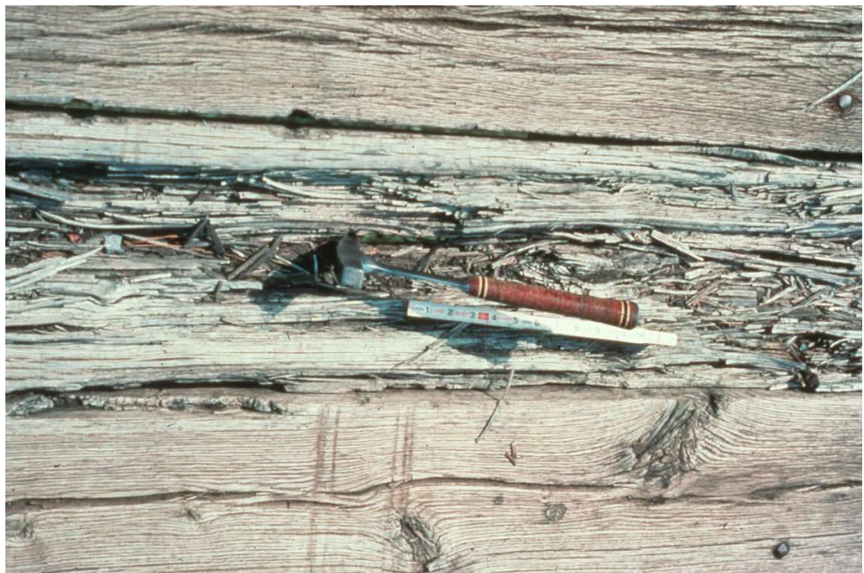
Figure 6.1.26 Weathering on Timber Deck
