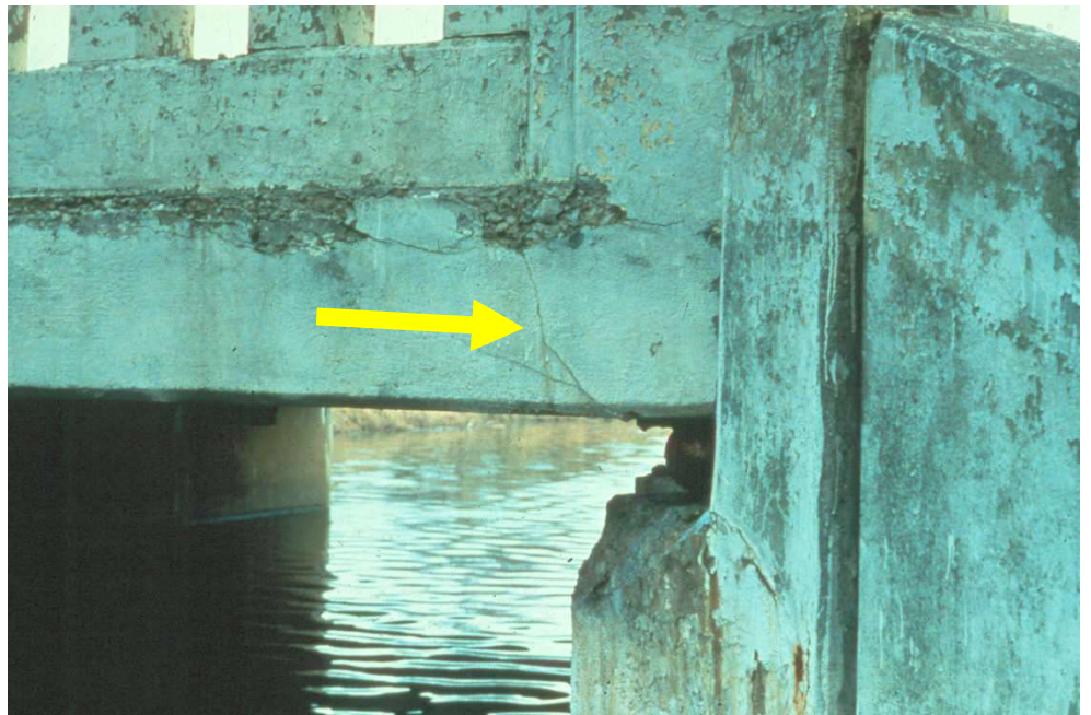
Figure 6.2.13 Shear Crack on a Slab
