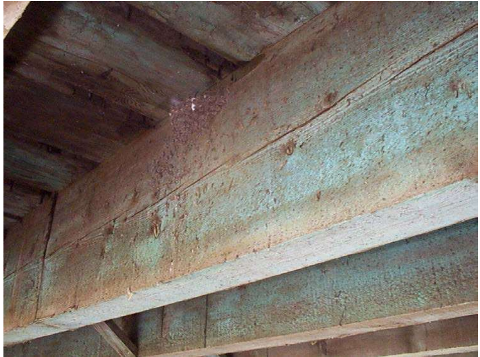
Figure 6.1.23 Horizontal Shear Failure in Timber Member
