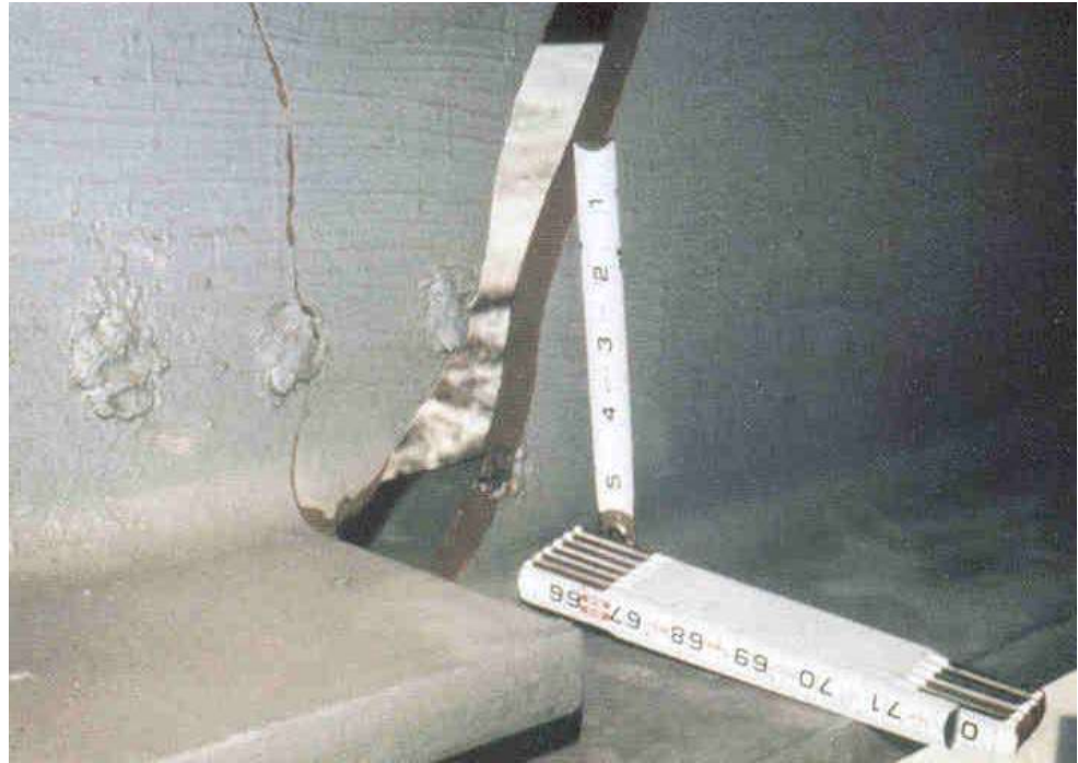
Figure 6.4.24 Crack Resulting from Plug Welded Holes
