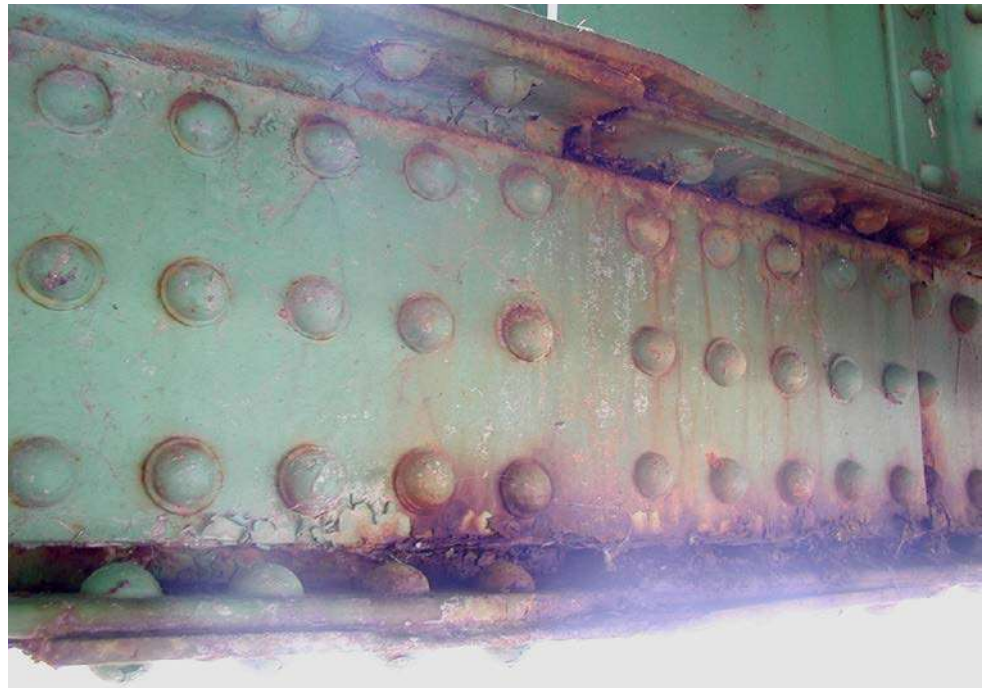
Figure 6.3.24 Corroding Rivet Head
