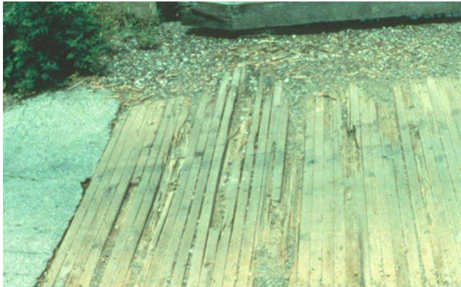
Figure 6.1.22 Wear of a Timber Deck
