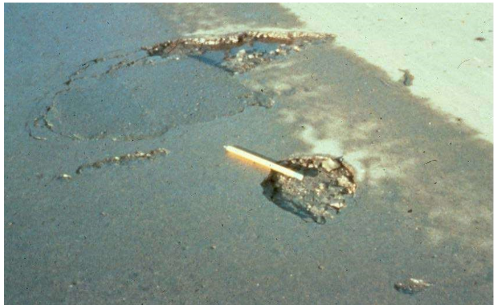
Figure 6.2.24 Spalling on a Concrete Deck
