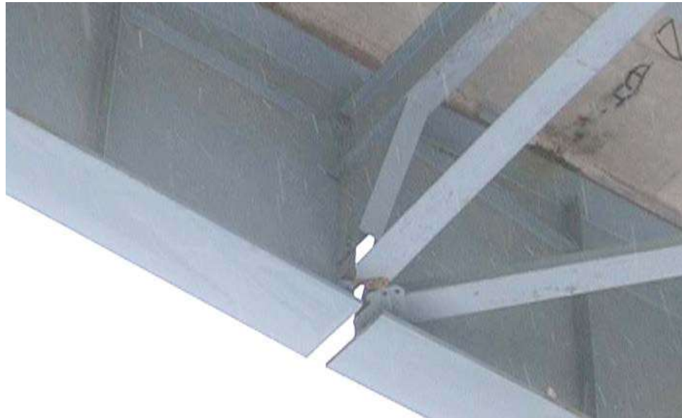
Figure 6.4.47 Local Triaxial Constraint Condition Resulting in Fracture on the Hoan Bridge, Milwaukee, Wisconsin
