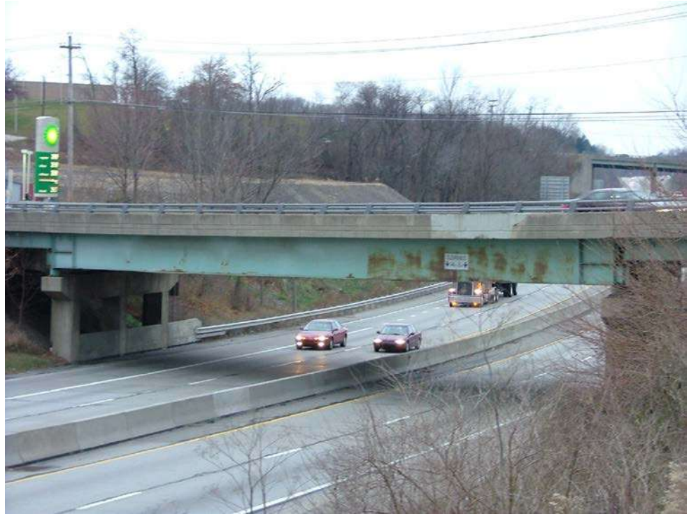
Figure 6.3.25 Roadway Spray Zone Deficiency
