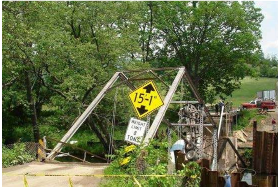
Figure 5.1.20 Damaged Bridge due to Failure to Comply with Bridge Posting
