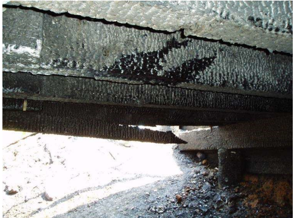
Figure 6.1.20 Fire Damaged Timber Members
