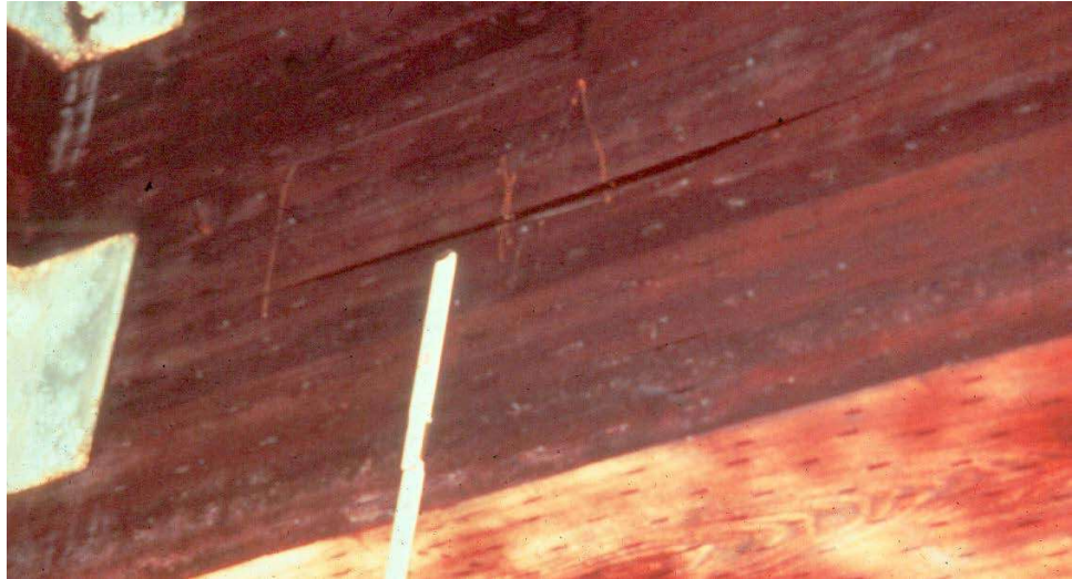
Figure 6.1.18 Delamination in a Glue Laminated Timber Member
