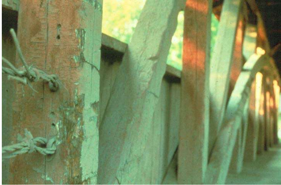
Figure 6.1.21 Impact/Collision Damage to a Timber Member
