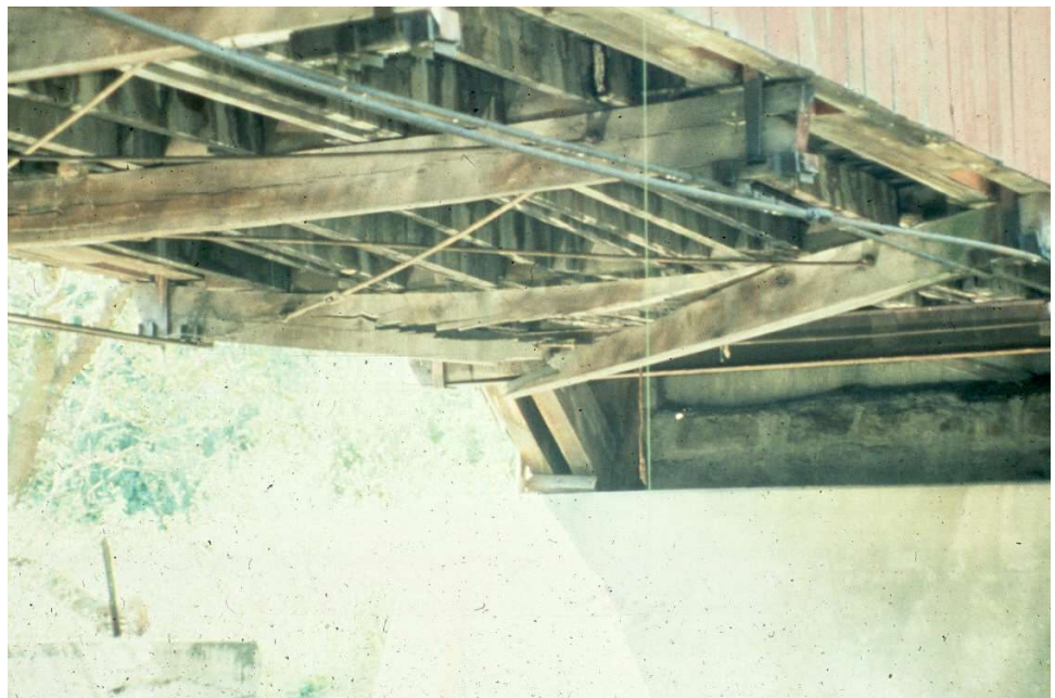
Figure 6.1.24 Failed Timber Floorbeam due to Excessive Bending Moment
