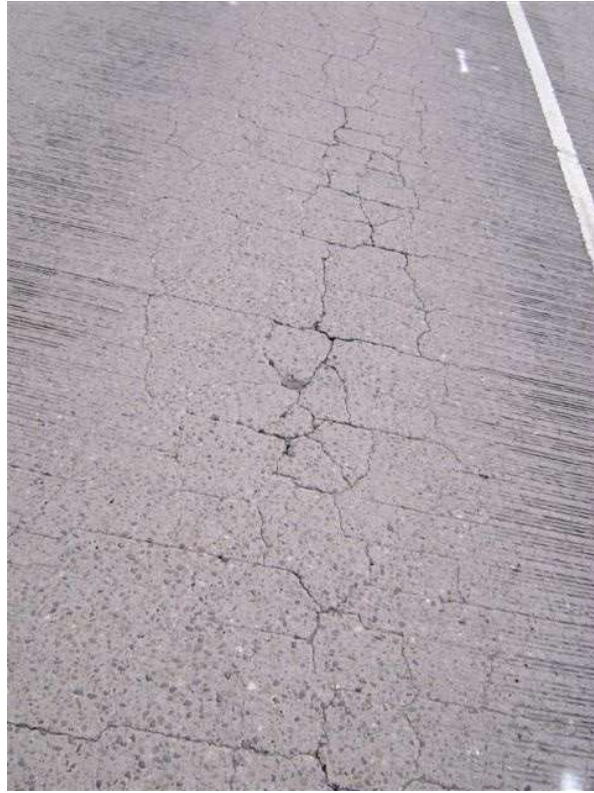
Figure 6.2.19 Pattern or Map Cracks
