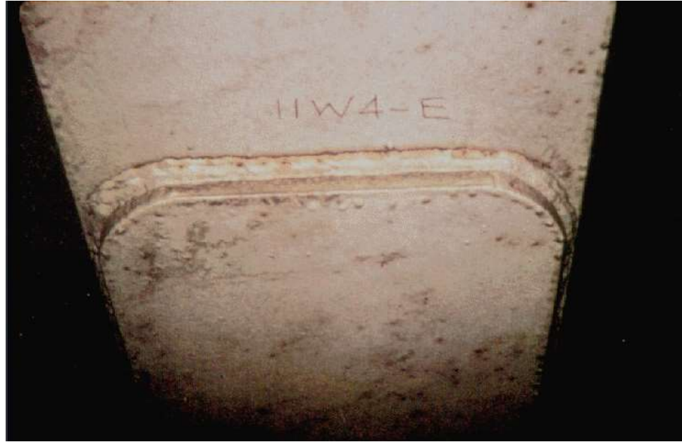
Figure 6.4.34 Part-Through Crack Growth at Cover Plate Welded to Flange
