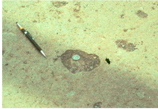
Figure 6.2.20 Light or Minor Scaling
