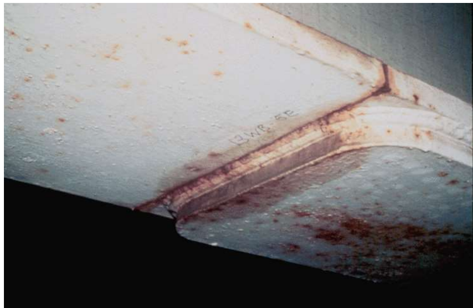
Figure 6.4.36 Through Crack at a Cover Plated Flange
