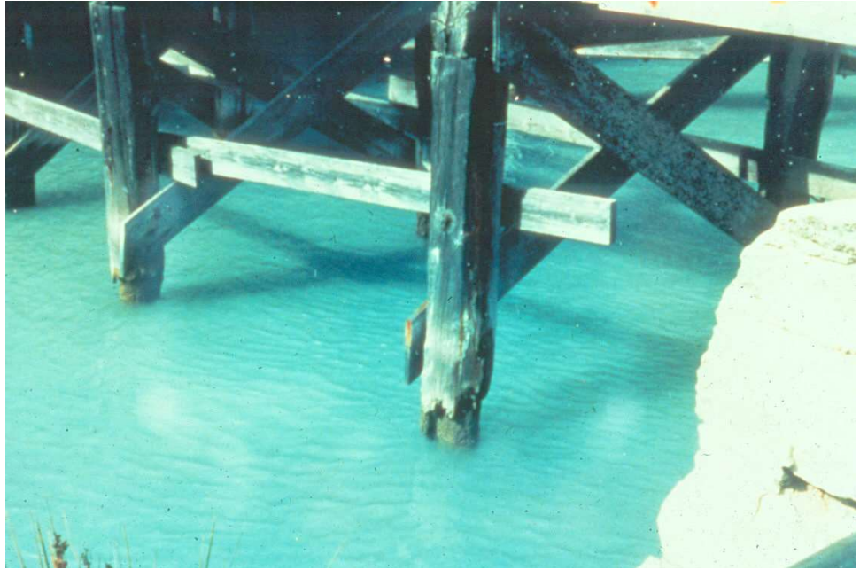
Figure 6.1.15 Marine Borer Damage to Wood Piling
