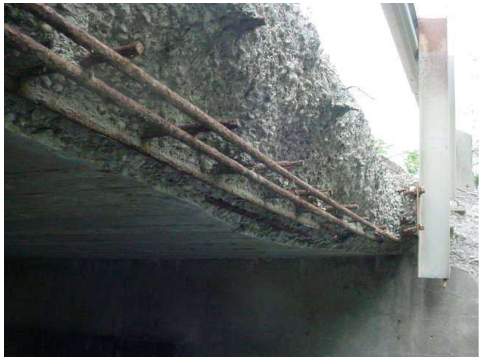
Figure 6.2.31 Loss of Bond: Concrete / Corroded Reinforcing Bar
