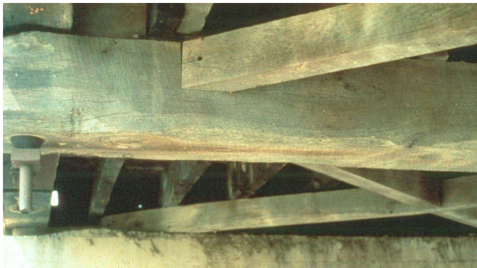
Figure 6.1.19 Loose Hanger Connection Between the Timber Truss and Floorbeam
