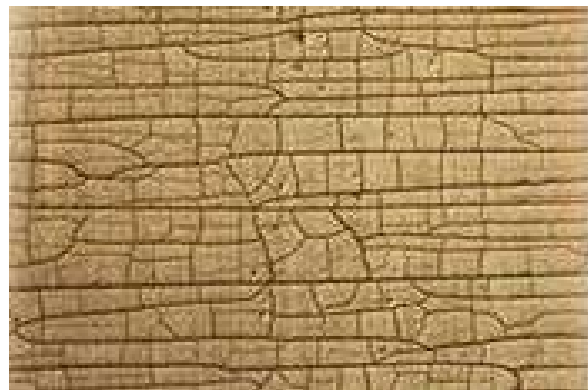
Figure 6.3.18 Paint Peeling from Steel Bridge Members
