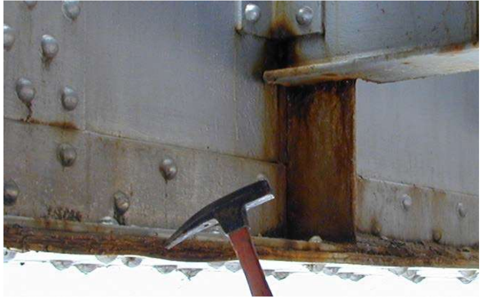
Figure 6.3.20 Corrosion of Steel
