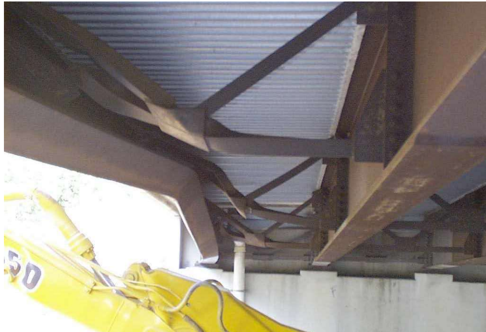
Figure 6.4.31 Severe Collision Damage on a Fascia Girder
