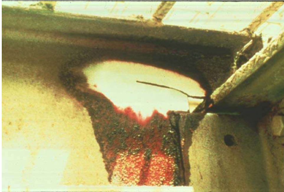
Figure 6.4.28 Crack Initiation at Coped Web in Stringer to Floorbeam
