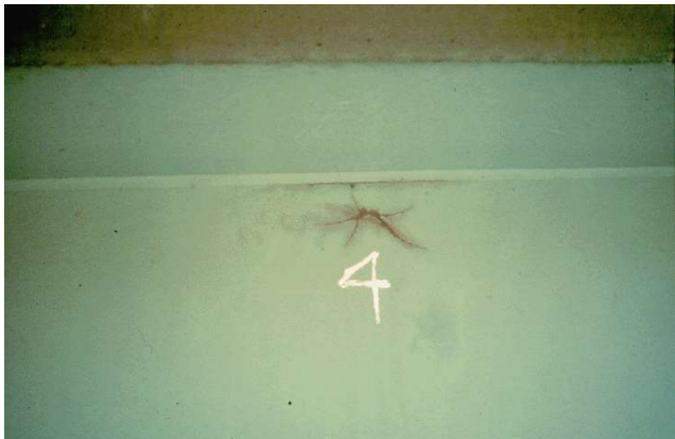
Figure 6.4.41 Through Crack in the Web
