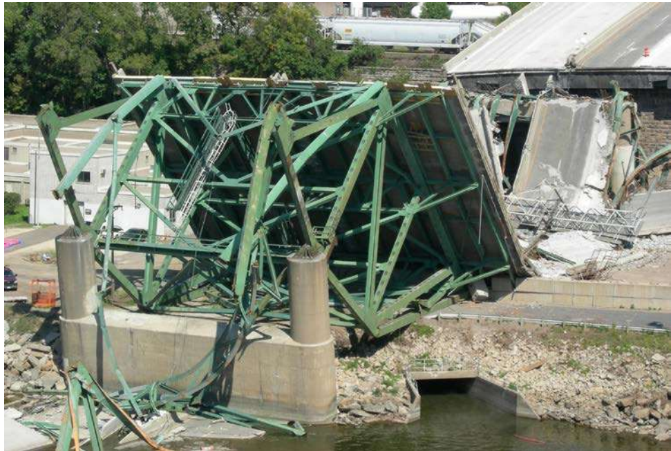
Figure 6.4.3 I-35W Mississippi River Bridge Collapse
