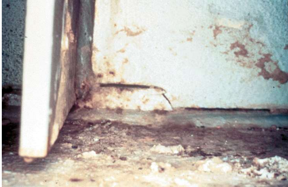
Figure 6.4.42 Through-Crack Ready to Propagate into the Flange
