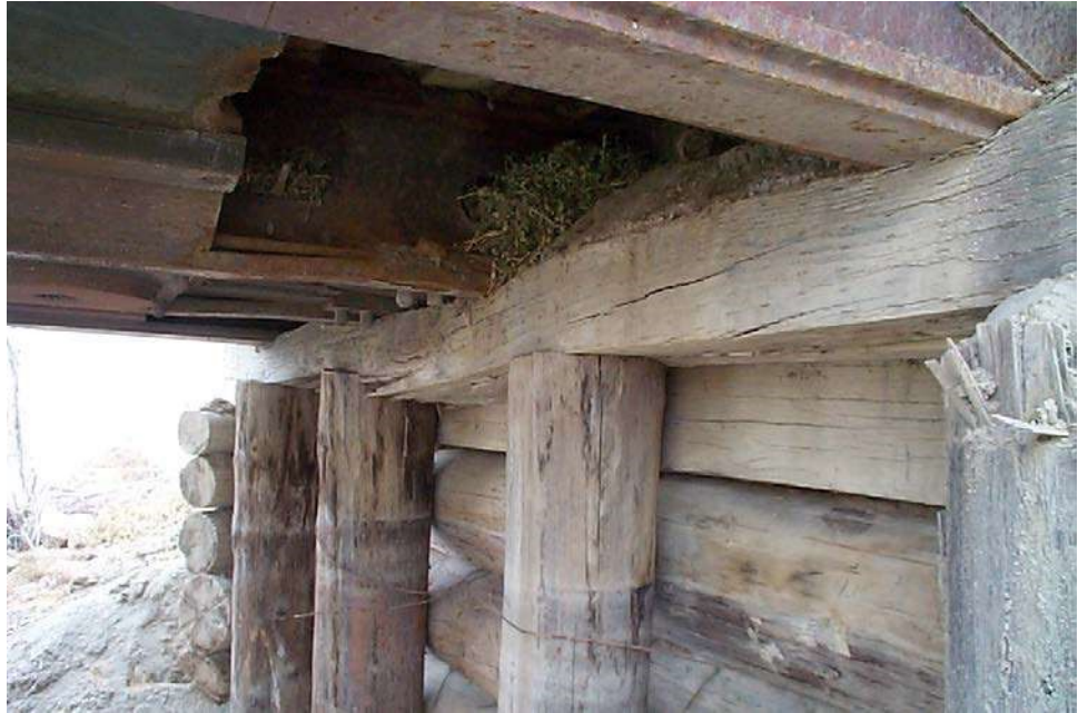
Figure 6.1.25 Timber Substructure Member Subjected to Crushing and Overstress
