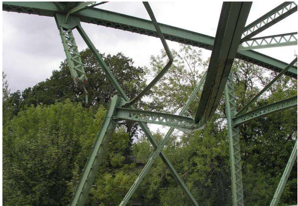
Figure 6.3.13 Collision Damage on a Steel Bridge
