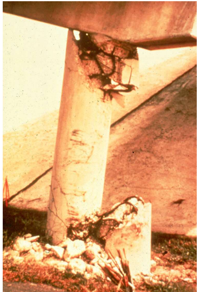
Figure 6.2.28 Concrete Column Collision Damage
