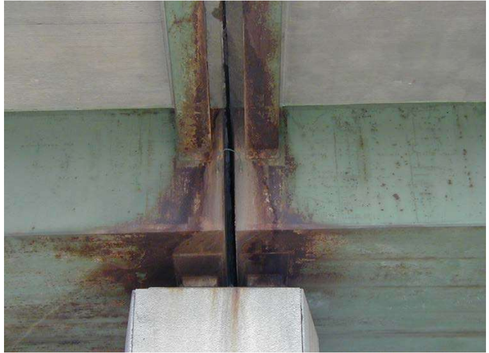
Figure 6.3.23 Water and Salt Runoff Near Expansion Joint
