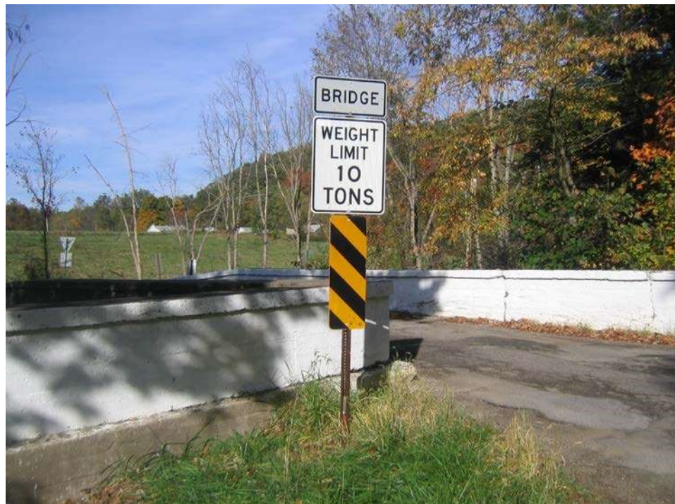
Figure 5.1.19 Bridge Weight Limit Posting
