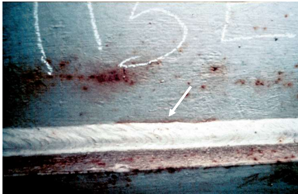
Figure 6.4.33 Part-Through Crack at a Cover Plated Flange
